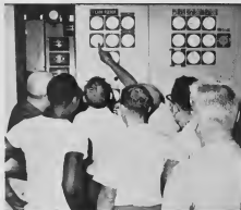
THE OBJECT of attention indicates voltage, and is being read to ascertain the correct functioning of the tap changing device on the transformers. The tie in of government electrical power took place Aug. 29.
